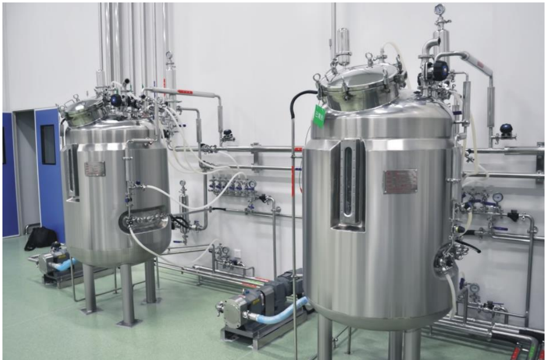
300L Storage tank
